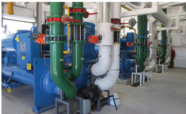
Chillers & Chilled Water Treatment Chemicals
